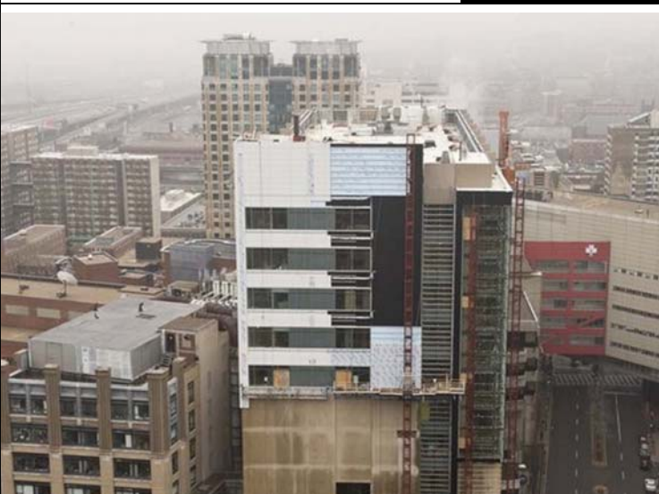
Aerial view of the vertical expansion project at Tufts Dental (Photo: http://dental.tufts.edu )
