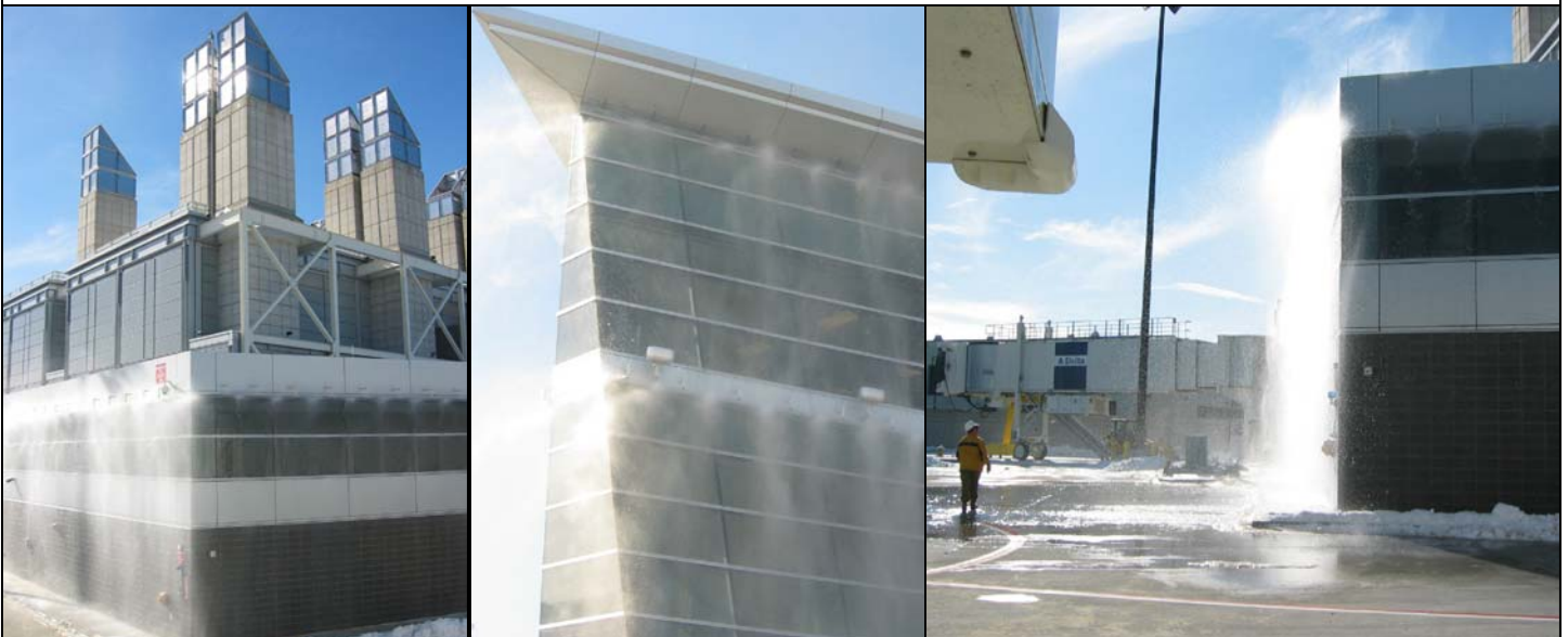
The deluge system suppresses the fire as designed. Photos show the deluged water from various angles.
