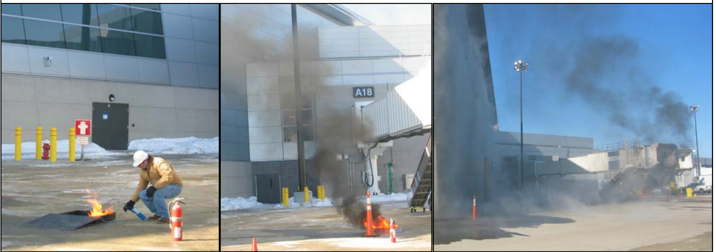
Once the system was installed, the testing began. A small fire and smoke surround the buildings at Terminal A.
