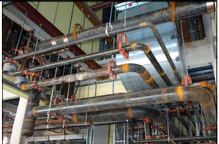
This intricate piping is installed in the building's first floor
