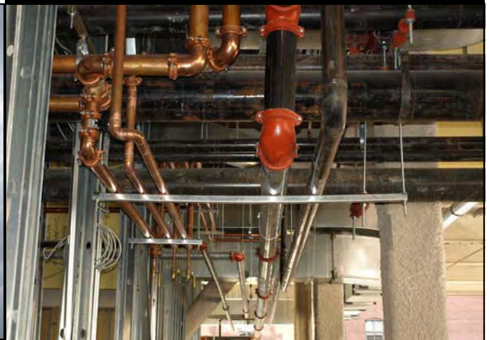
From the fab shop to the job site, the pipe is set in place
