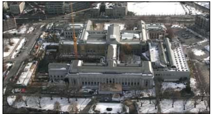
Aerial view of the construction site at the MFA Boston. - Photo courtesy of www.mfa.org .
